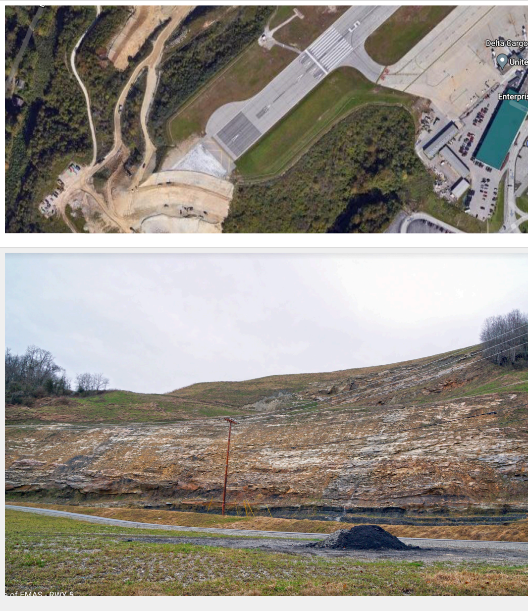
Figure 1. Charleston (West Virginia ) Airport Runway 5 end after geotechnical collapse of retention wall.
